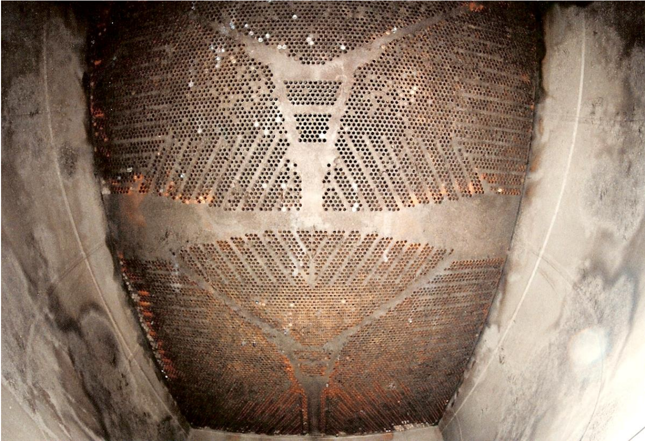
End view of the cooling water tubes in a condenser
